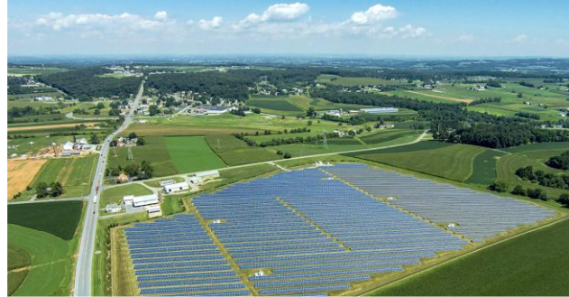
3 MW Merchant Generator
